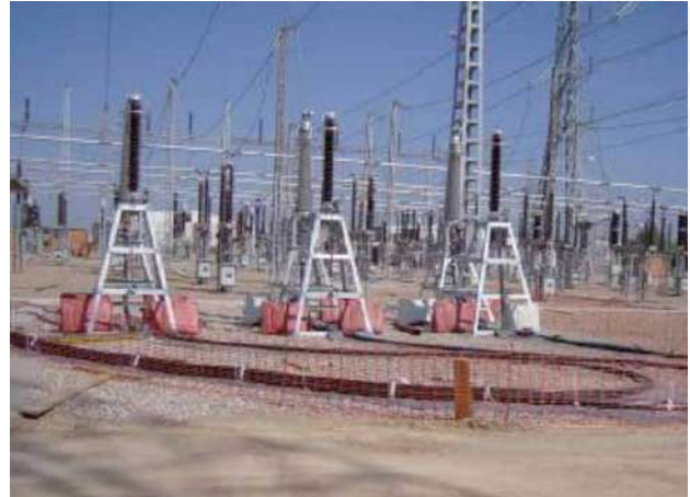
Typical use of stand-by link far maintenance in substations
