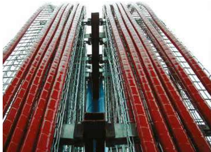
Example of more space busy by cable tray distribution
